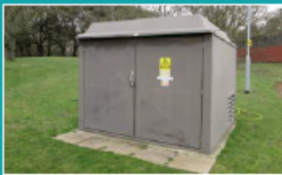
Example of a typical substation that serves residential/commercial properties with electricity
